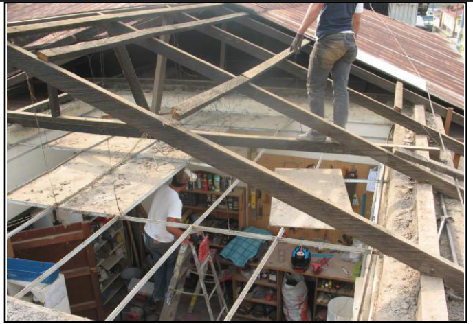
Nicaraguan workers, funded by ISLA, completed a major re-roofing and re-ceiling of the Jalapa war veterans center and storage areas this spring.
